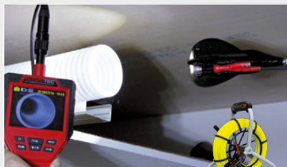
Ventilation inspection and servicing
