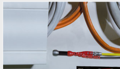
Shafts and underfloor ducting
